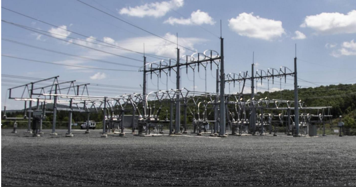
COMPARABLE SUBSTATION PHOTO
