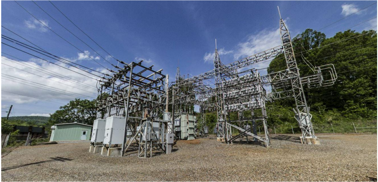
EXISTING STUART RETIREMENT SUBSTATION
