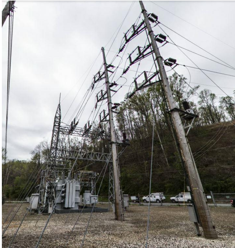
EXISTING BASSETT RETIREMENT SUBSTATION
