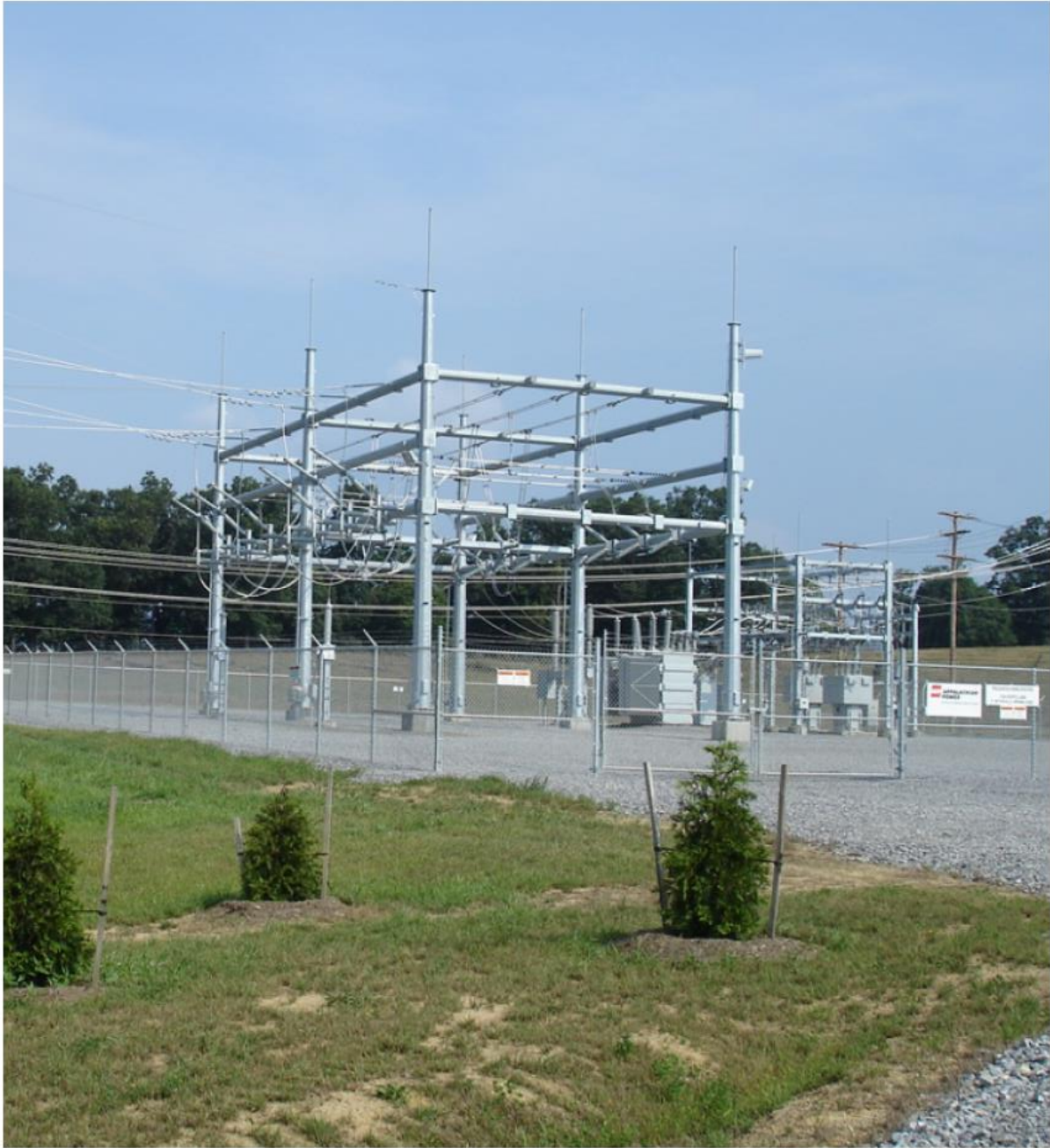
COMPARABLE SUBSTATION PHOTO
