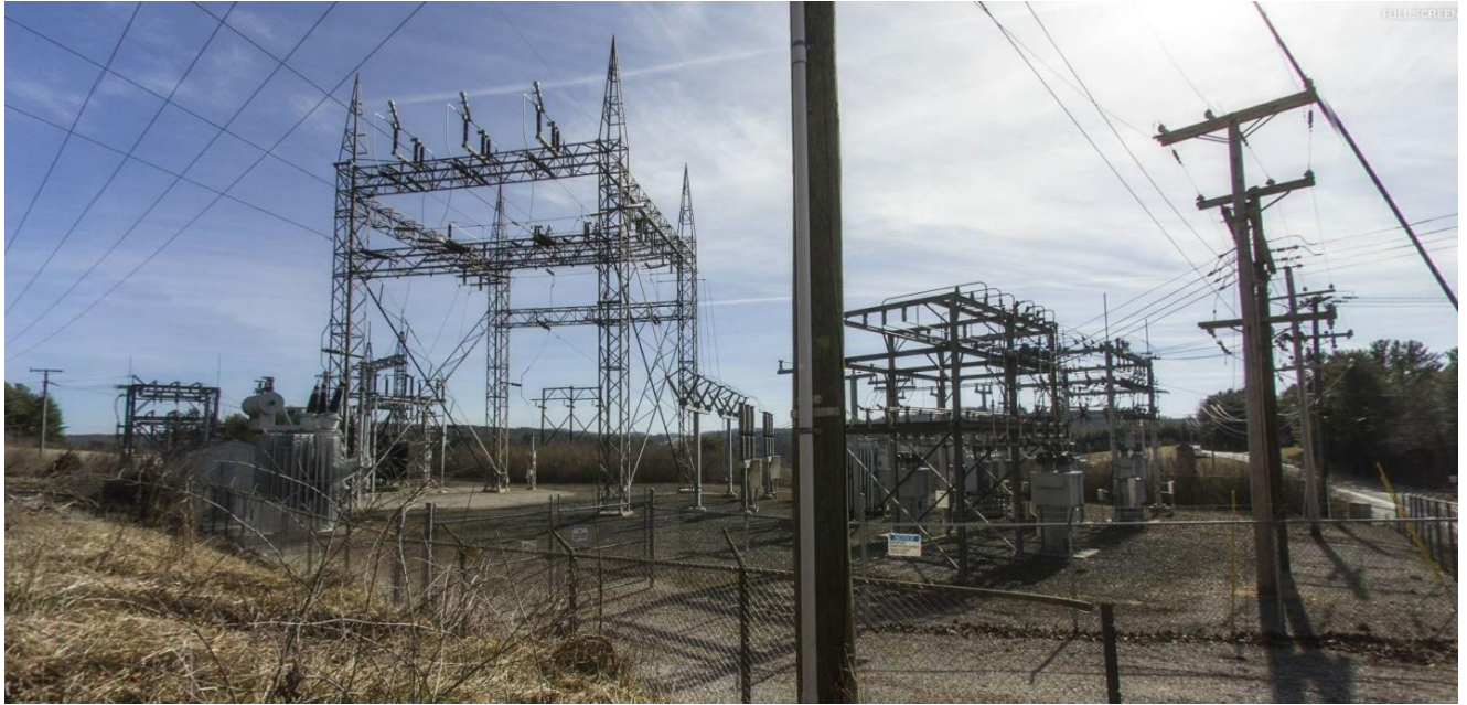
EXISTING FLOYD SUBSTATION
