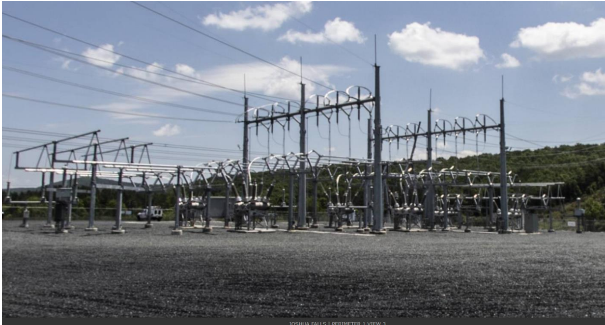
JOSHUA FALLS | PERIMETER 1 VIEW 3 COMPARABLE SUBSTATION PHOTO
