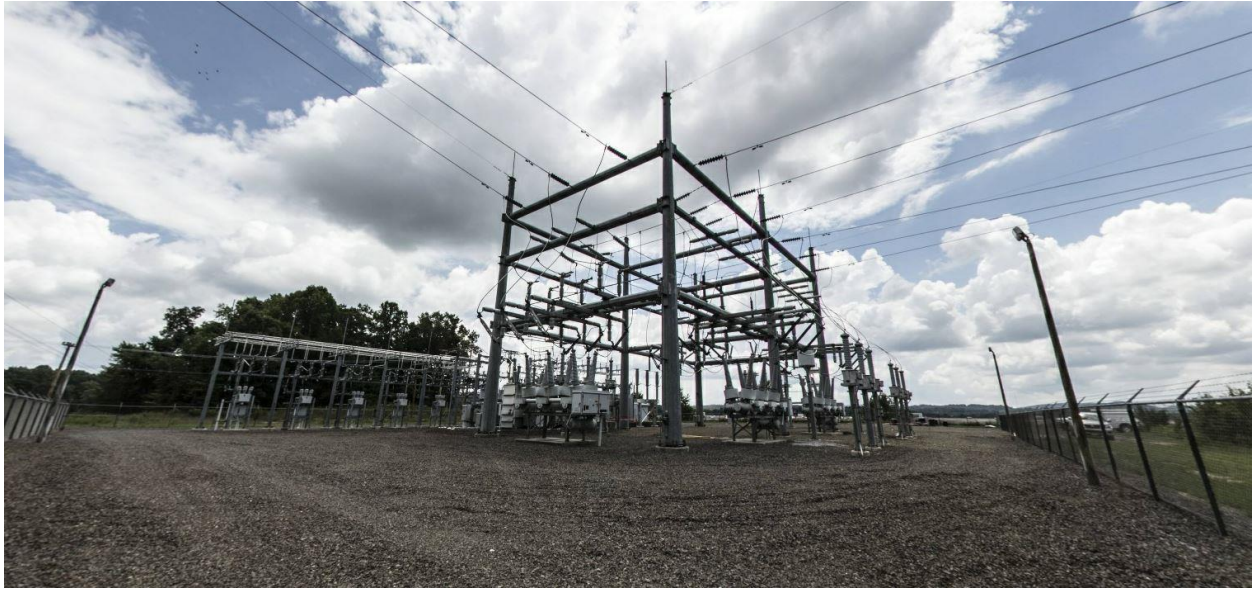
EXISTING HUFFMAN SUBSTATION
