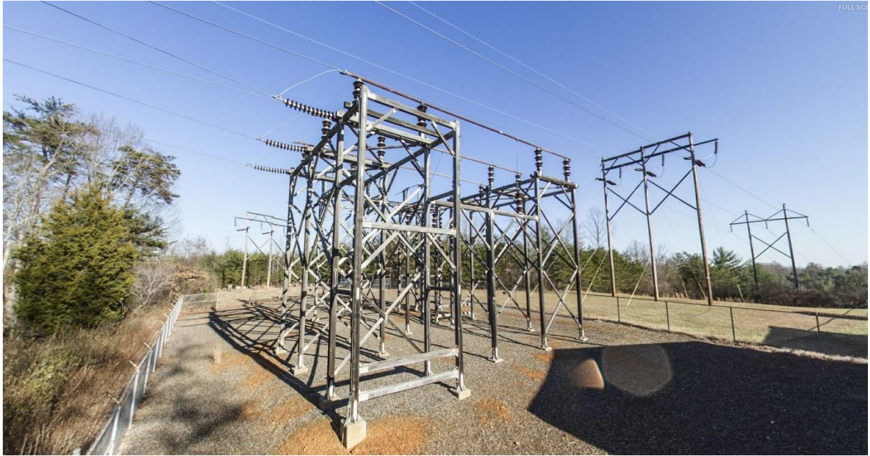
EXISTING PHILPOTT SWITCH SUBSTATION (to be Retired)
