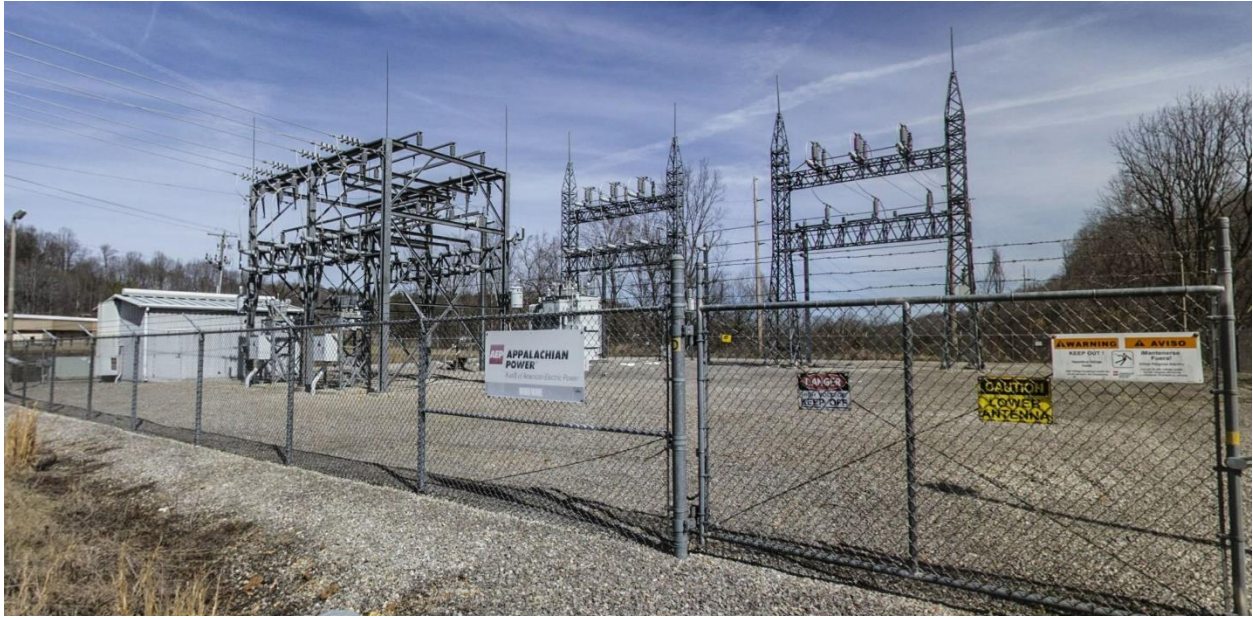
EXISTING WOOLWINE SUBSTATION
