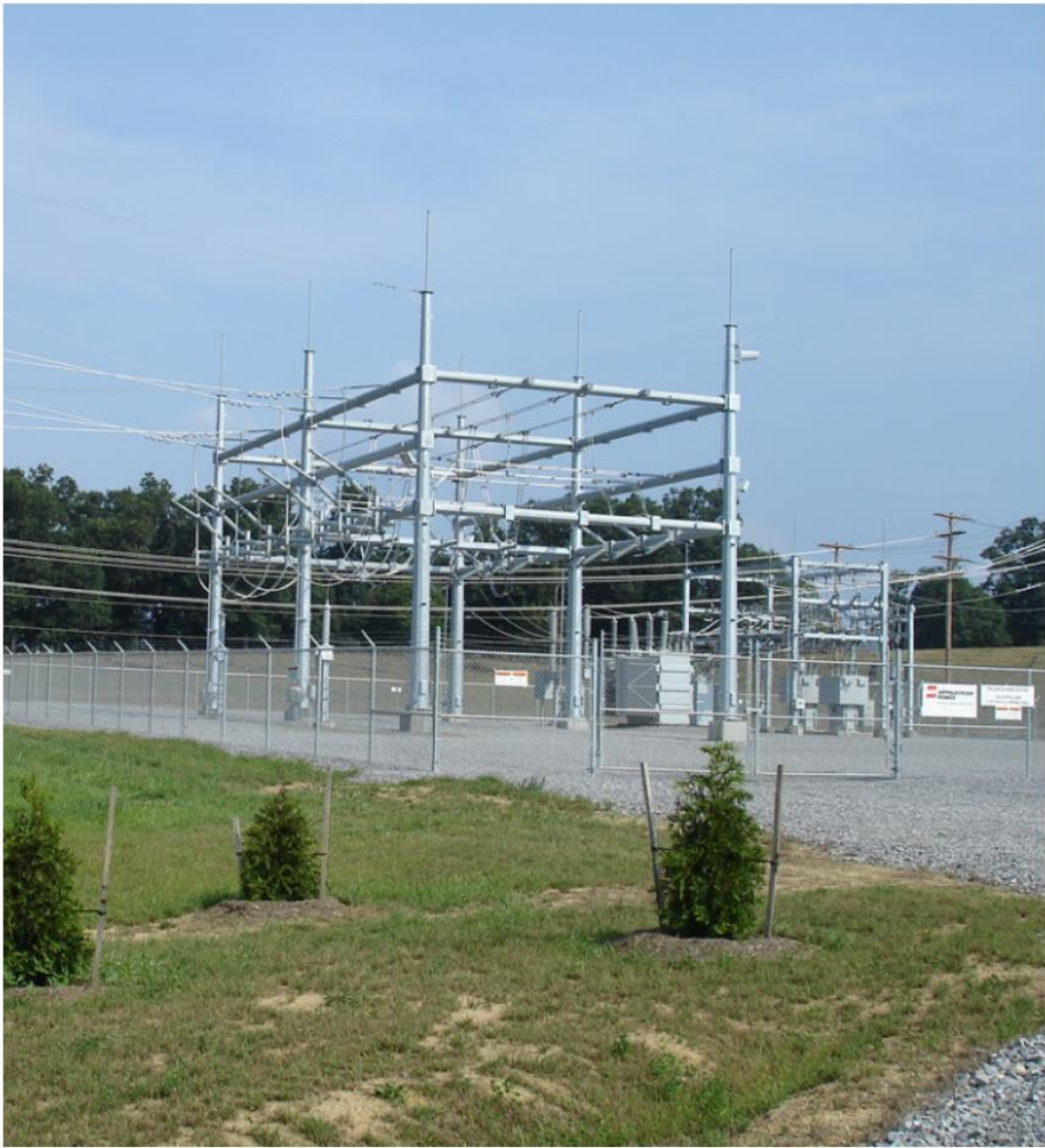
COMPARABLE SUBSTATION PHOTO
