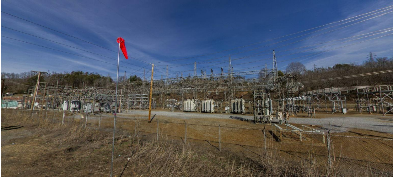
EXISTING FIELDALE SUBSTATION
