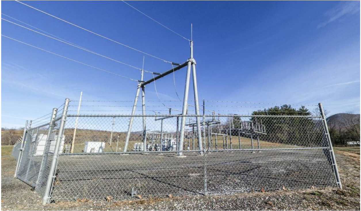
EXISTING WILLIS GAP SUBSTATION
