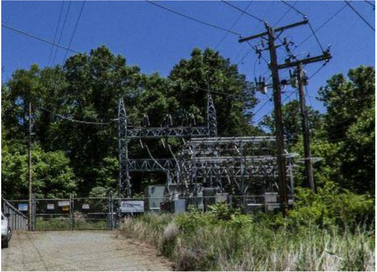
EXISTING STANLEYTOWN RETIREMENT SUBSTATION
