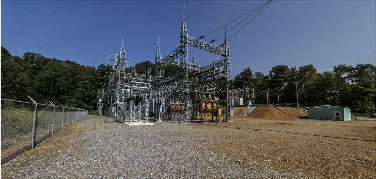
EXISTING WEST BASSETT RETIREMENT SUBSTATION
